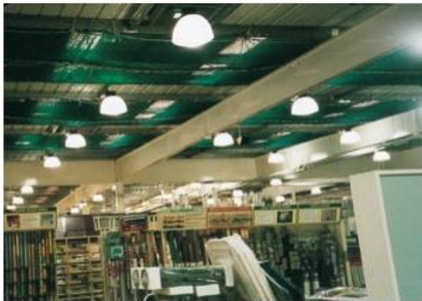
Safety netting used to provide protection for roof lights during minor roof works
