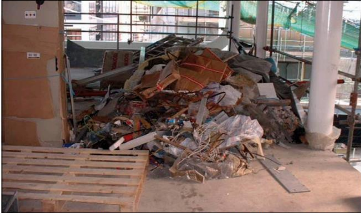
Figure 6 Most construction rubbish can burn. Make sure that it is swept up and removed from the site as soon as possible
