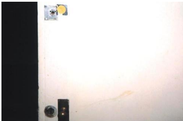
Figure c Painted asbestos insulating board facing to a fire door with some damage around the door furniture
