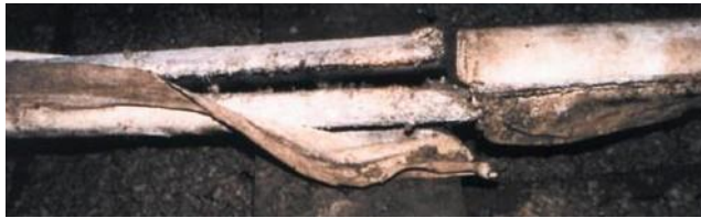
Figure a Asbestos-insulated water pipes showing evidence of maintenance work damage, with detached preformed sections and calico wrapping
