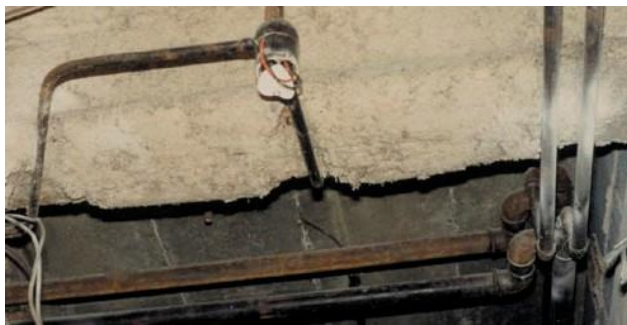
Figure b Poorly tamped sprayed chrysotile fireproofing on a structural steel beam holding up a concrete floor, showing some overspray onto the concrete and damage by electrical work
