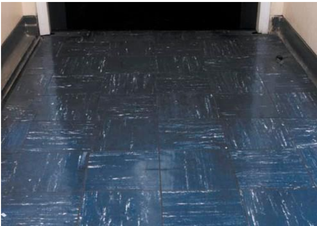
Figure e Asbestos-containing vinyl floor tiles
