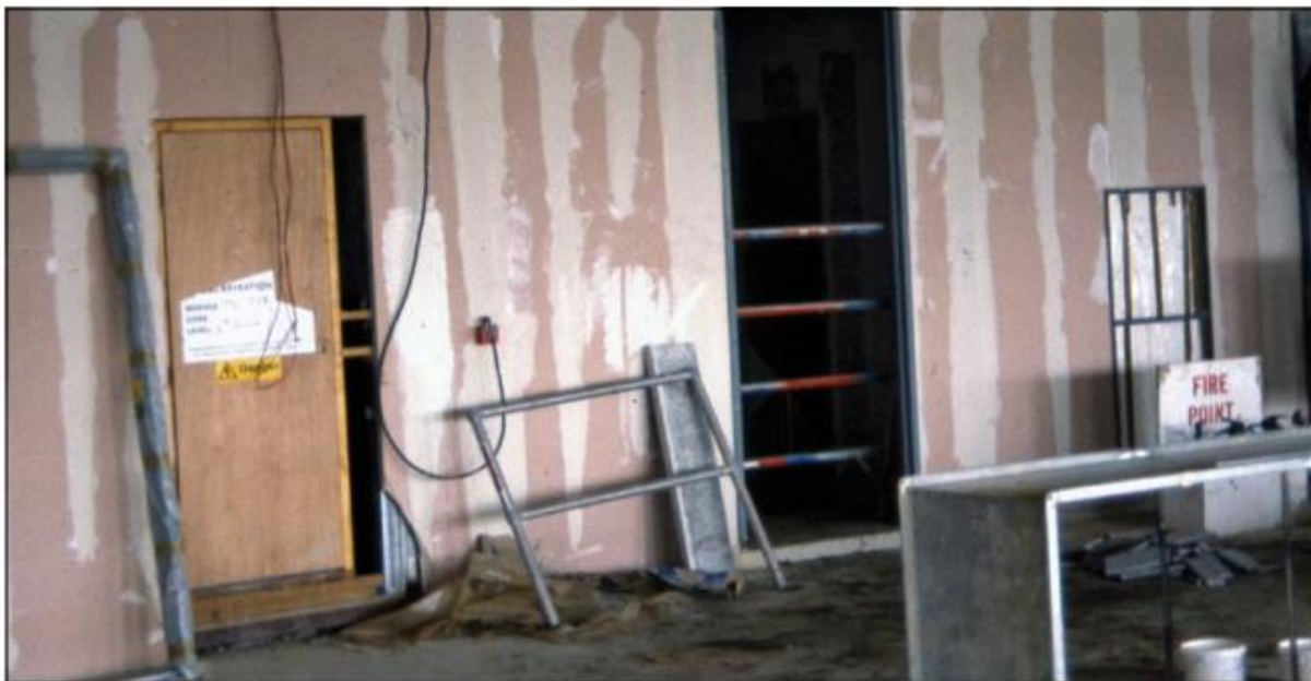
Figure 14 Plasterboard partitions such as this can form effective compartmentation. It is important that all gaps are filled in. In this case, there are holes in the top of the partition and service ducts in the side rooms that need to be sealed
