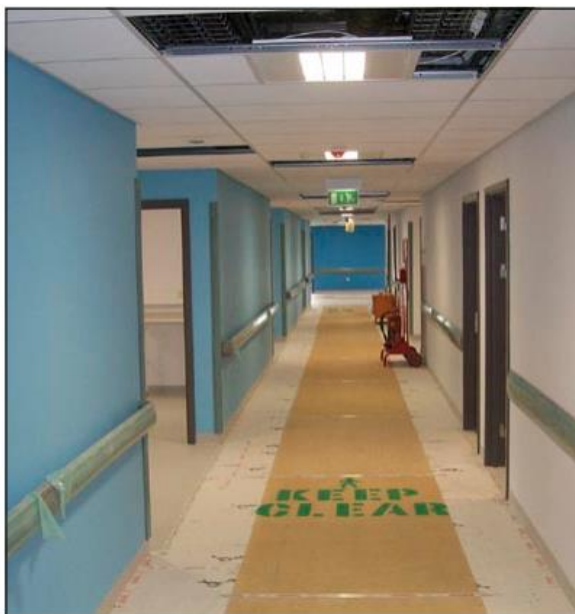
Figure 8(a) Keep fire exits clearly signed and free from obstructions
