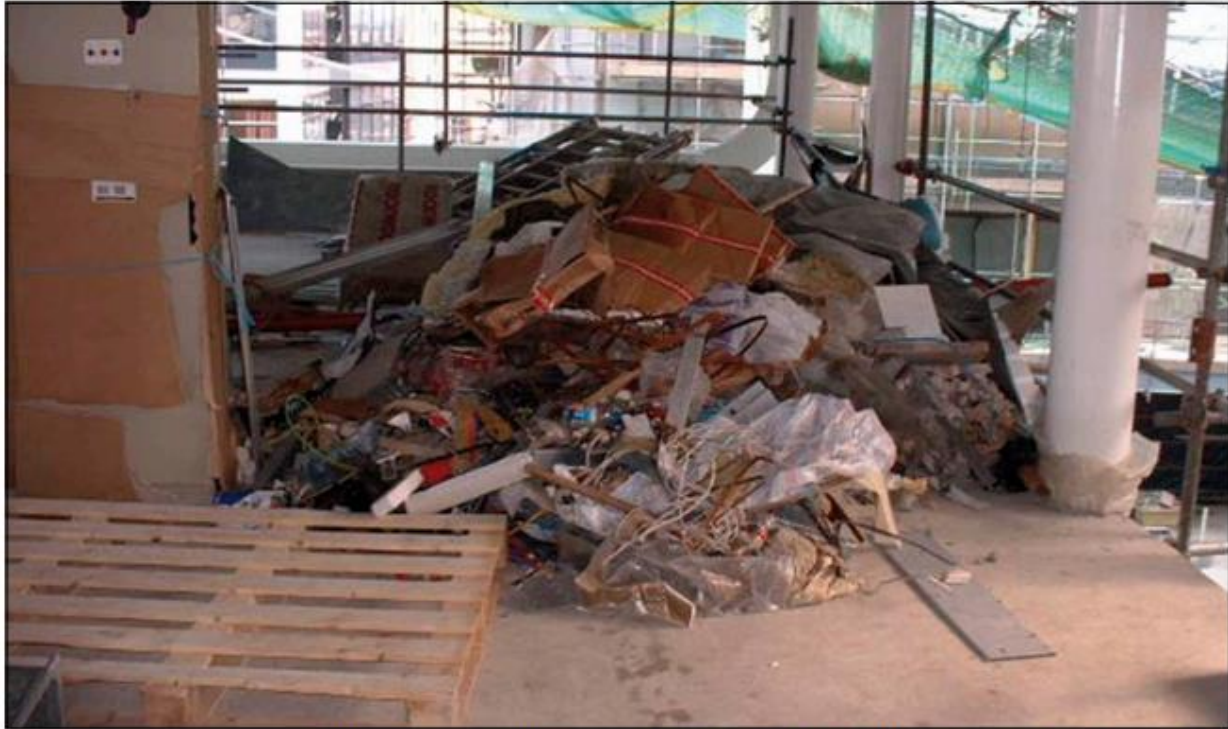
Figure 6 Most construction rubbish can burn. Make sure that it is swept up and removed from the site as soon as possible
