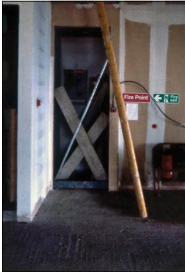
Figure 7 Avoid creating dead-ends and misleading fire exit signage
