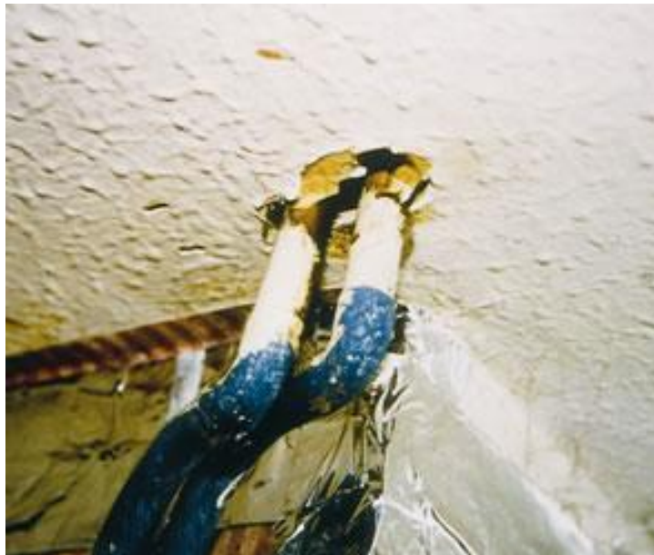
Damaged asbestos textured coating around pipework
