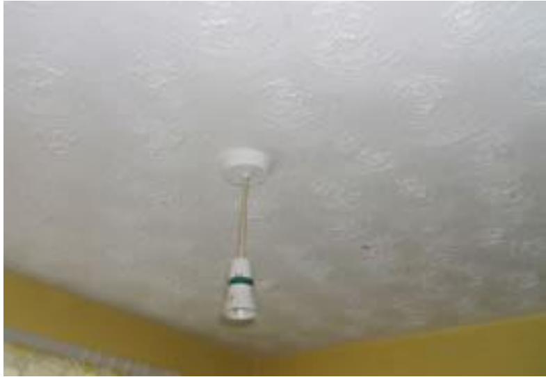
Asbestos textured coating (artex) on ceiling
