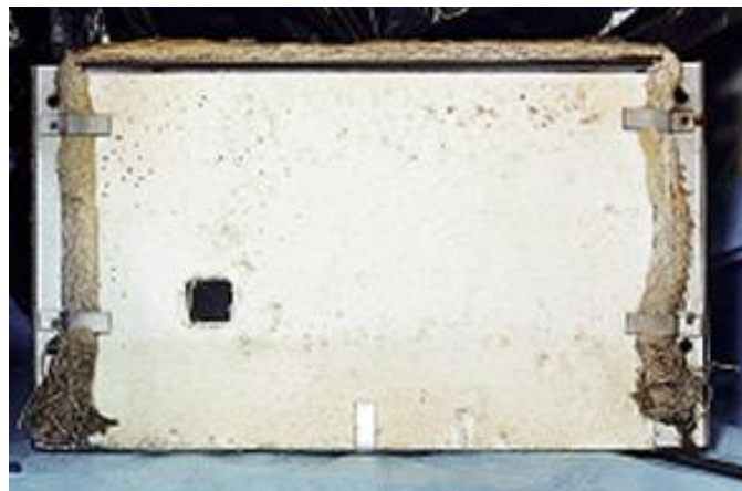
Asbestos rope seal on boiler
