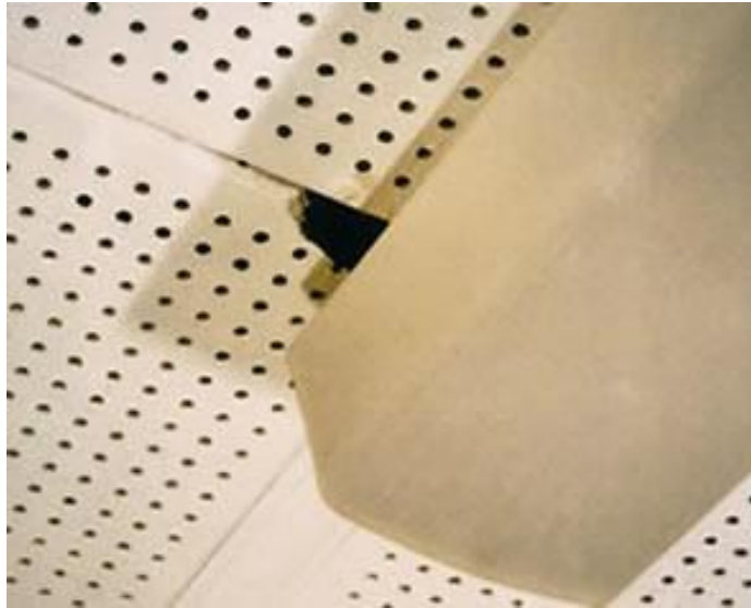
Damaged perforated ceiling tile
