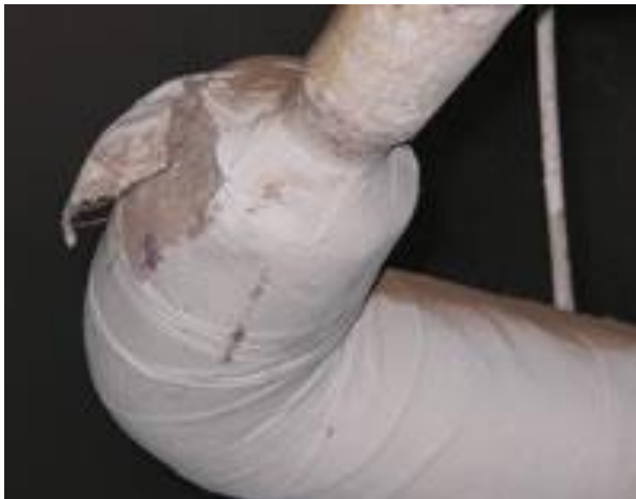
Damaged asbestos pipe Lagging
