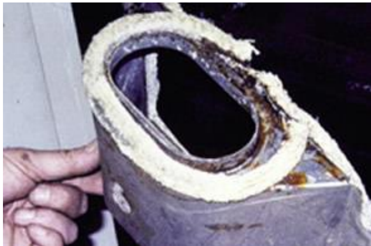
Asbestos rope seal on boiler
