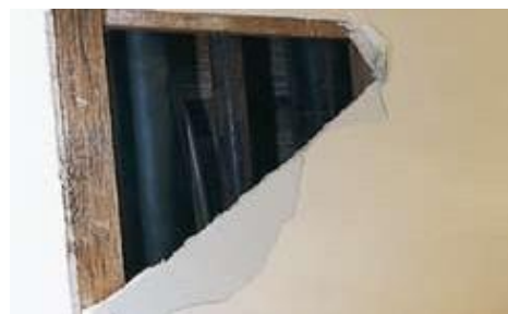
Asbestos insulating board (AIB)
